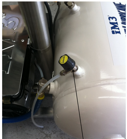
Compressor tank drain, located on-top of white air tank— open slowly Place container under white tube to collect water.
